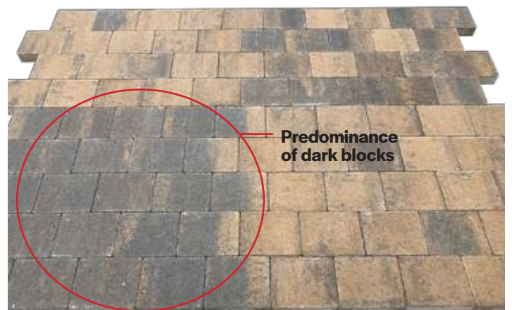
Image 6 - Example of poorly blended blocks
