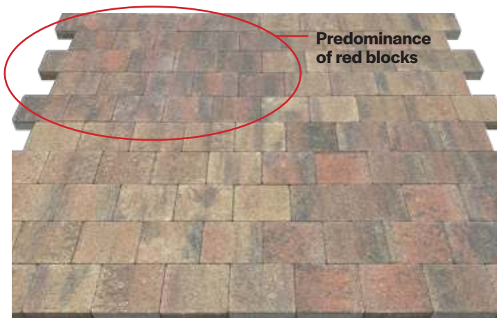
Image 5 - Example of poorly blended blocks
