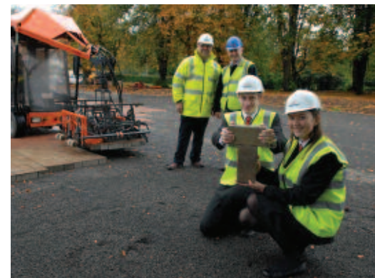
Pioneering Project – Tobermore's Hydropave system collects rainfall and stores the water in a specially designed sub base before releasing it very slowly into the schools neighbouring drainage systems. Hydropave was machine laid by Gibson Contracts in order to cut the costs of the project.
