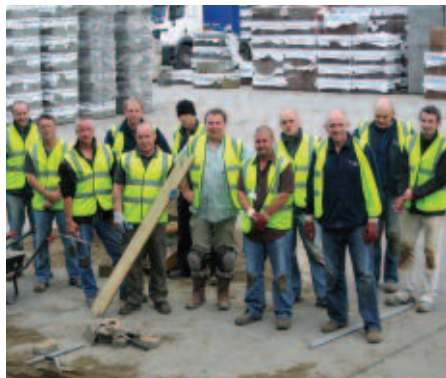
Tony McCormack pictured with some of the layers who took part in the Hard Landscape Training Group (HLTG), block paving installation course which was held recently at Tobermore headquarters.
