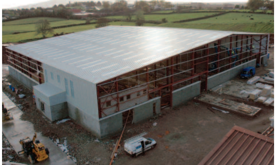
The construction of the new 3,500sqm manufacturing facility to house a new state-of-the-art block paving machine is already underway.
