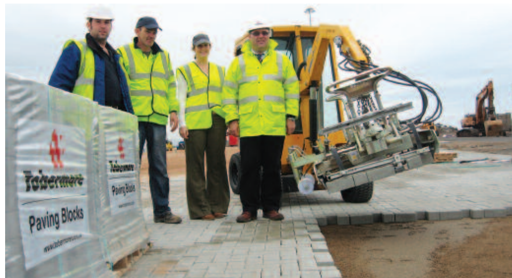
Jumping Port - R-L: Tobermore's Harry Badger pictured with Catherine Higgins and Brendan Kearns of Marmic Construction and Hamilton Walker, FP McCann at the new Victoria Dock at the entrance to Belfast Lough where 70,000 square metres of Tobermore's Pedesta paving is being laid by machine because of the very tight timescale for the project.
