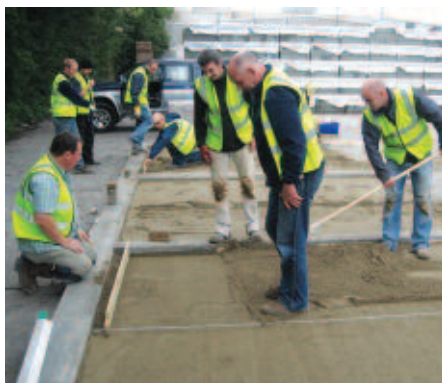
Tony McCormack passes on his wealth of expertise to paving contractors at the HLTG training at Tobermore.
