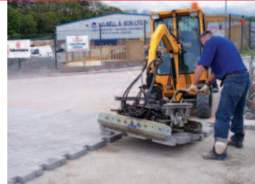
Ballywalter's NG Bell and Sons recently machine laid their massive 3,500 square metre yard on the Greyabbey Road in Tobermore's popular Pedesta paving. The speed with which the task was completed and the fabulous finished result, has had a big impact on the many customers who use this busy yard.
